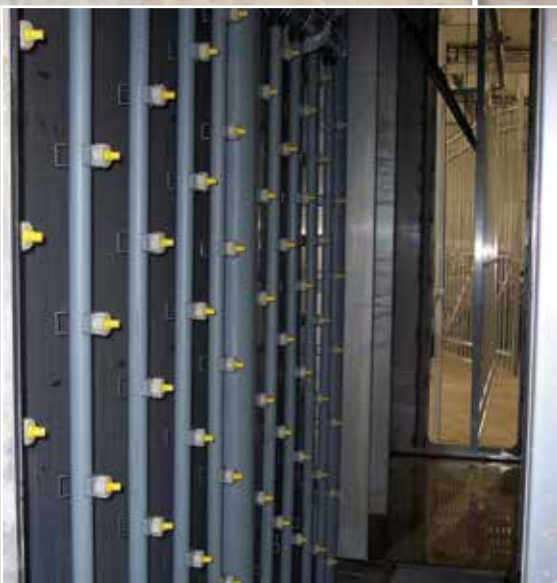
STEP #2: Product enters heated acidic cleaner stage to remove extrusion and fabrication oils.
