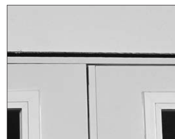
Figure 18: The gap between the door slabs and the head is not evenly aligned.
